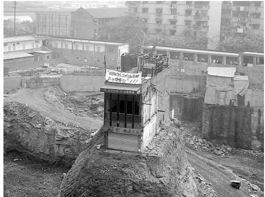
The owners of this "nail house" refused to obey an eviction order, thwarting plans for a shopping mall. (© Zhou Shuguang)
